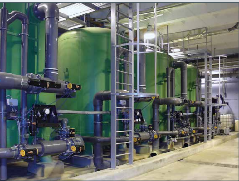
Continuous-flow adsorber in a water treatment plant
