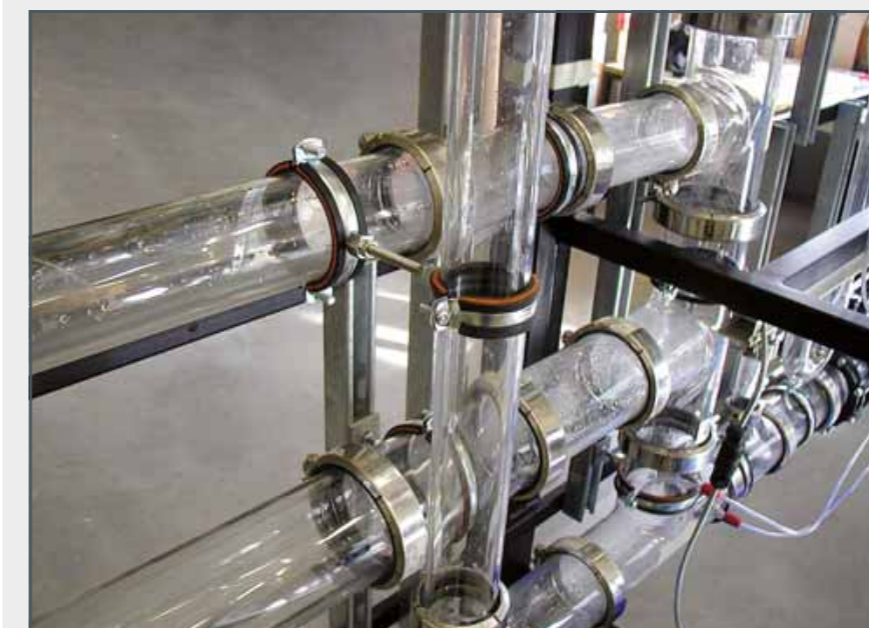
Pipes and valves and fittings made of glass
