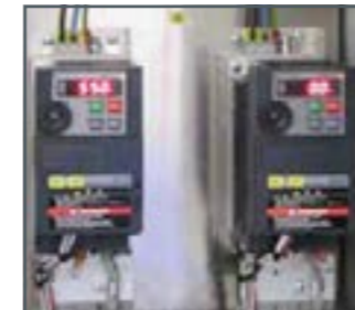
Frequency converters for controlling the pumps
